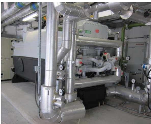
Figure 10.22 An adsorption chiller
