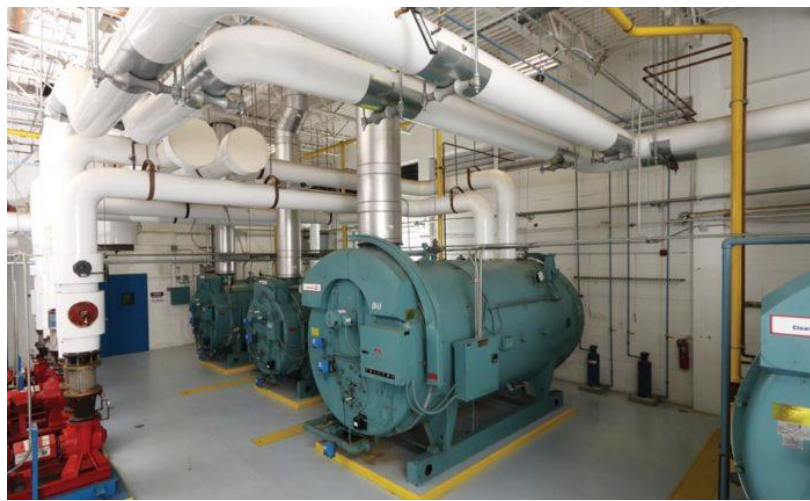
Boilers in a central heating plant
