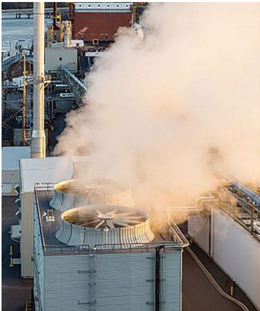
Figure 6.24 White plume emitted by cooling towers
