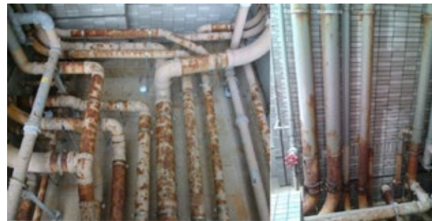
Pre-mature rusting of cast iron pipe without proper access for inspection and maintenance
