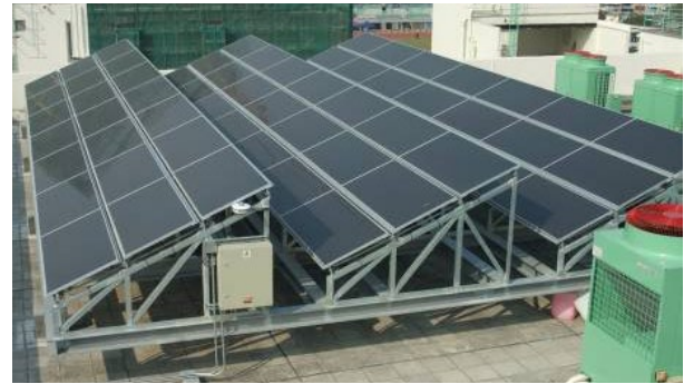
A grid-connected PV system installed on a school building roof
