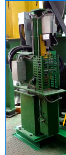
Overspeed governor & pit diverter pulley for lower car
