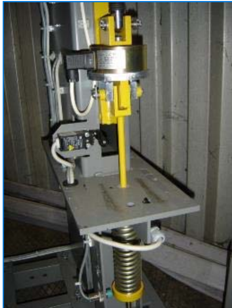
Motor with solenoid in upper end position S191: safety circuit closed
